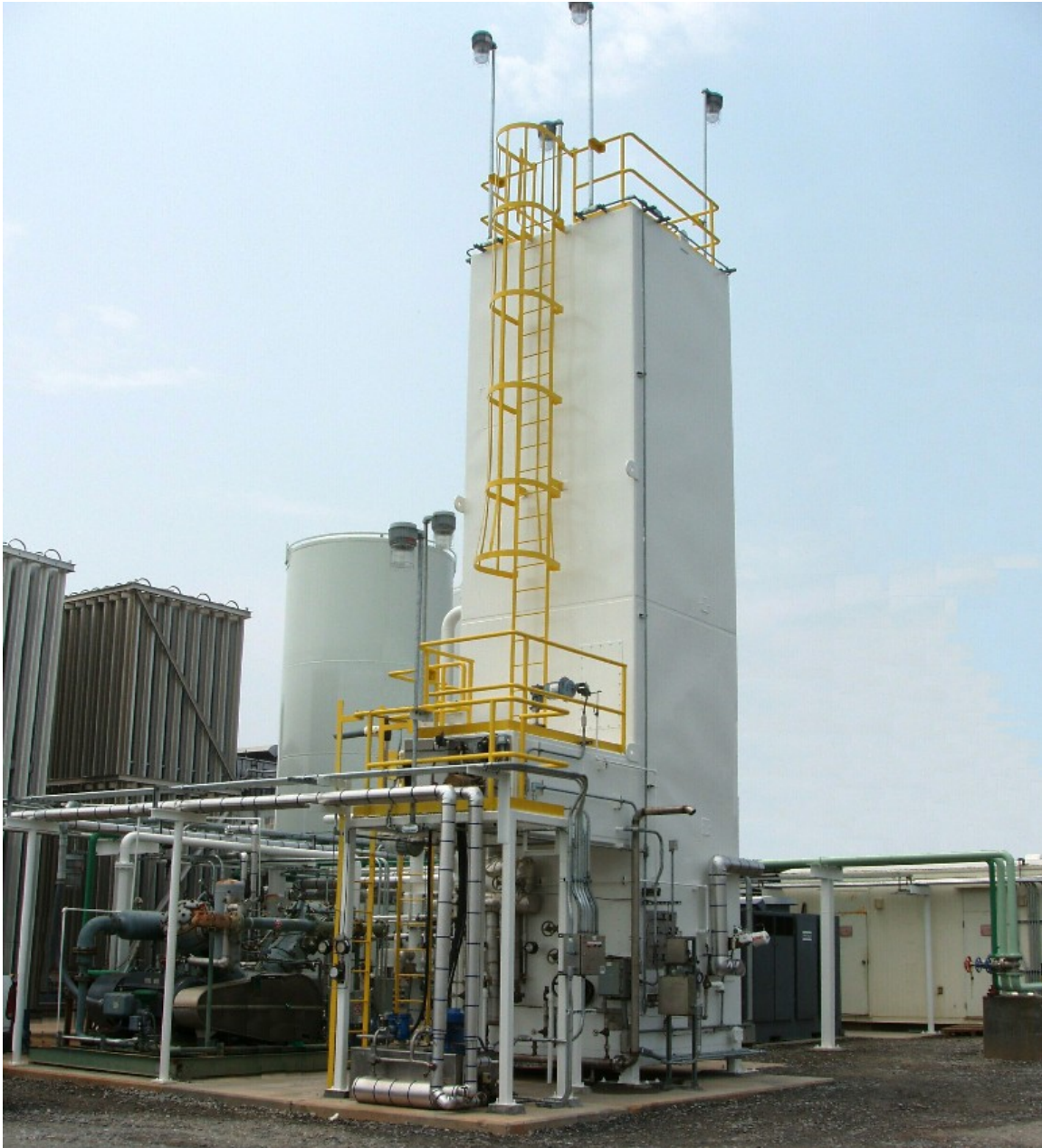
Universal Cryo Gas nitrogen generator in North Carolina Product Compressor, Cold Box and Air Compressor.
