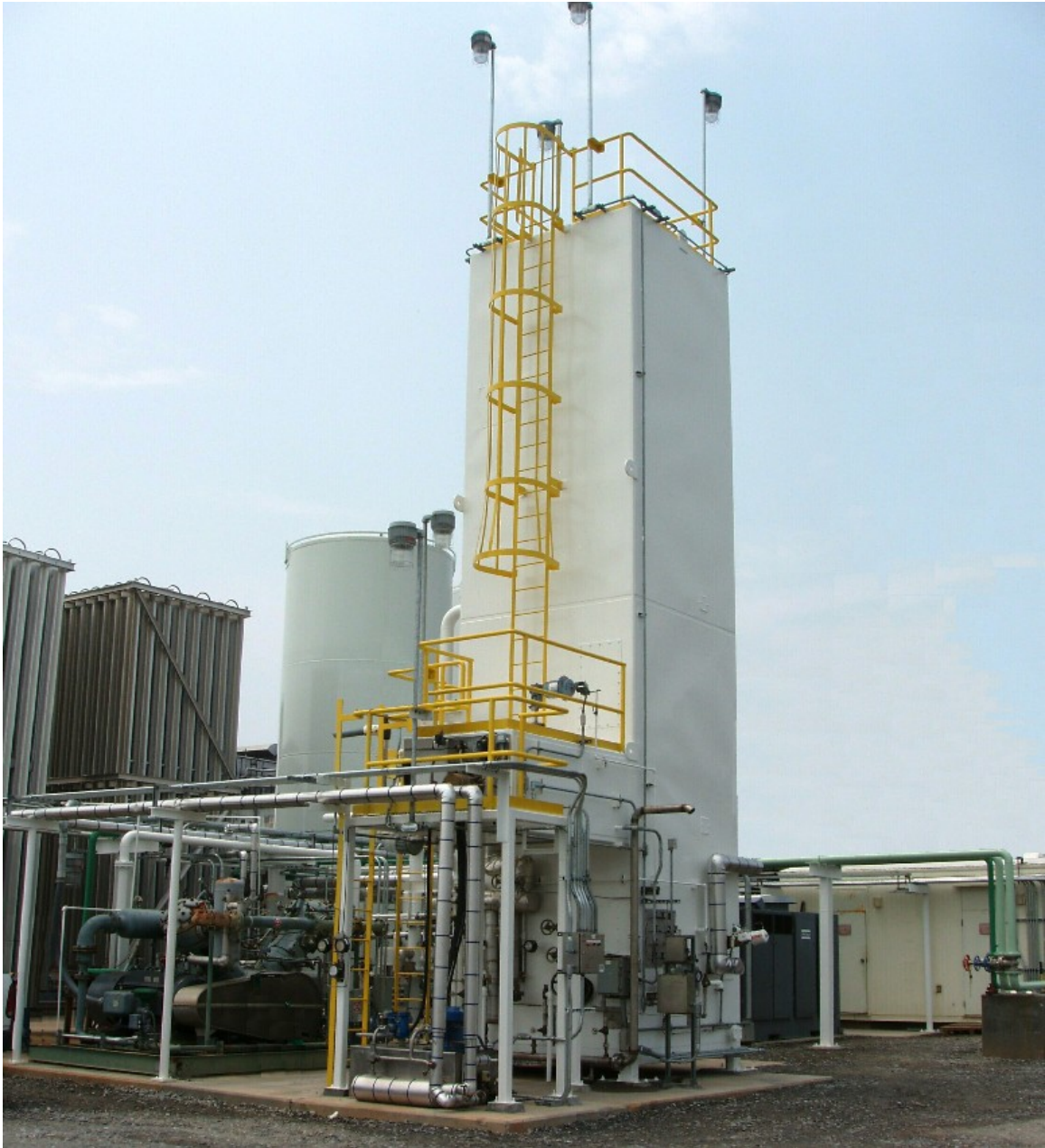
Universal Cryo Gas nitrogen generator in North Carolina Product Compressor, Cold Box and Air Compressor.
